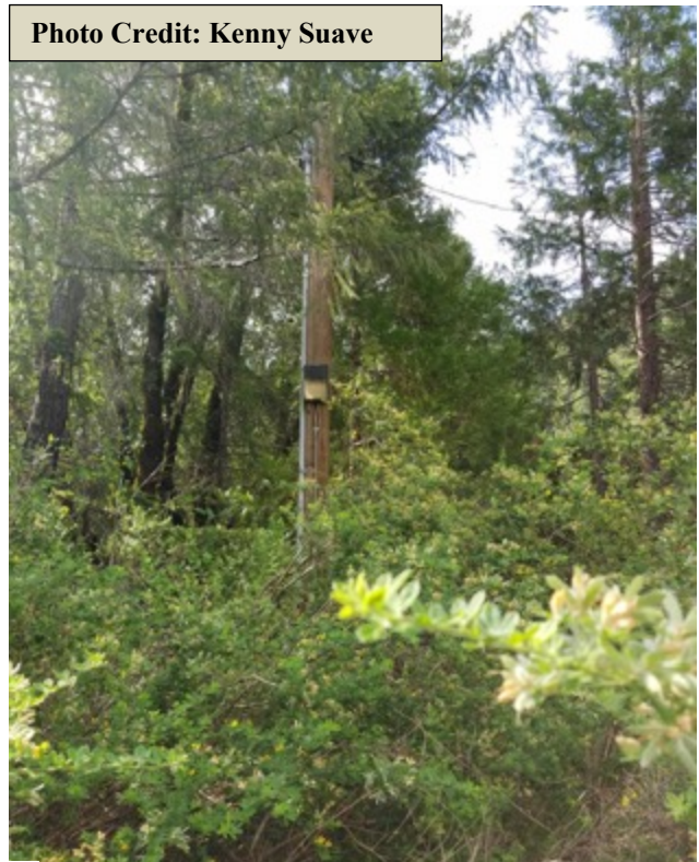
Figure 5.4 Power pole in Corridor Needing Maintenance
